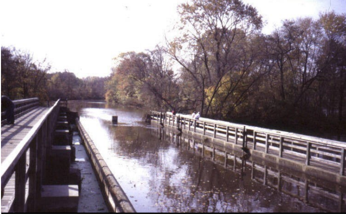
The Millstone Aqueduct carries the canal over the Millstone River in Plainsboro, off Mapleton Road.
