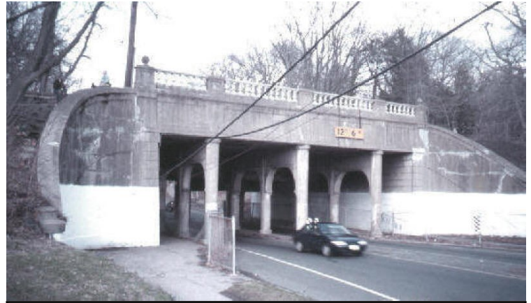
The canal and the railroad were carried over Parkside Avenue in Trenton by this aqueduct.
